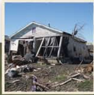
Historic home damaged by Hurricane Katrina in New Orleans.
